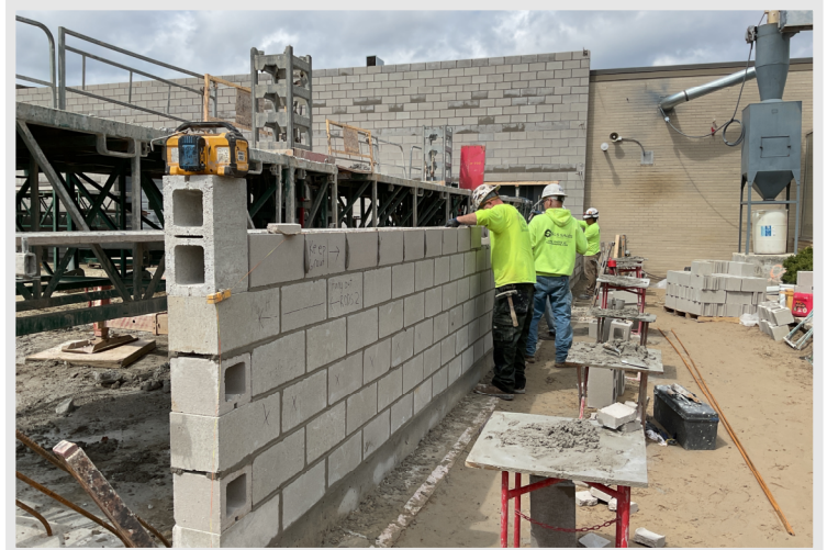
Findorff masons working to build the load-bearing masonry walls at the Skills Lab Addition. Structural steel erection will follow once complete.
